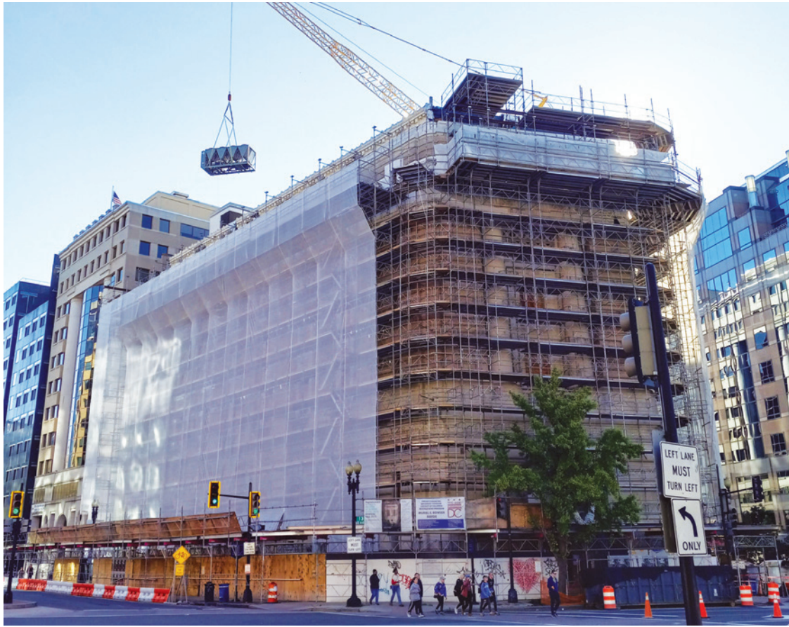
In early October, a construction crane hoists new chiller equipment up to its rooftop destination.
